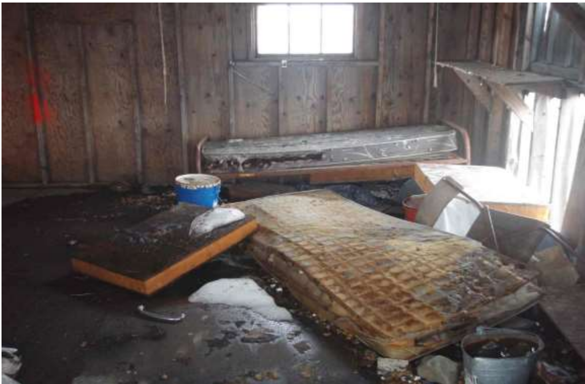
Figure 28: General debris and waste found inside buildings on site WB-9, June 2012
