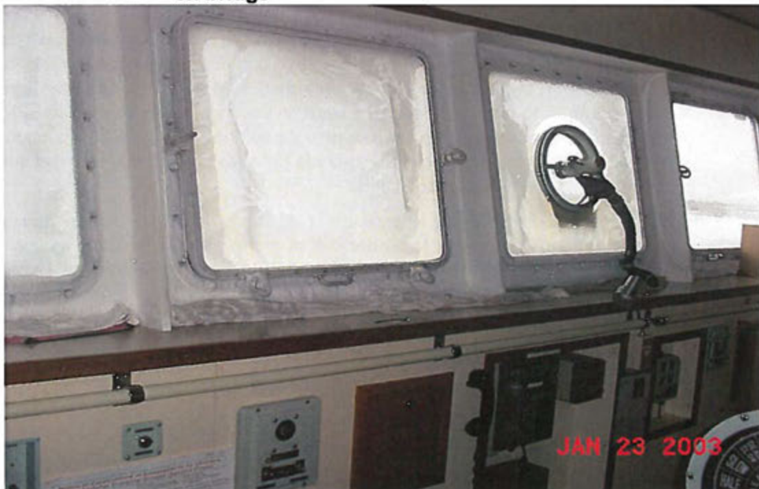
Figures 9.1B – Deficient wheelhouse heating combined with a high rate of humidity
