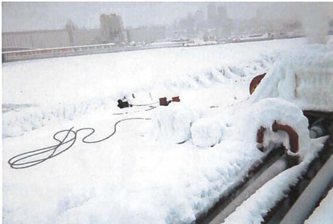
Figures 5.3F– Deck, piping and valves inaccessible
