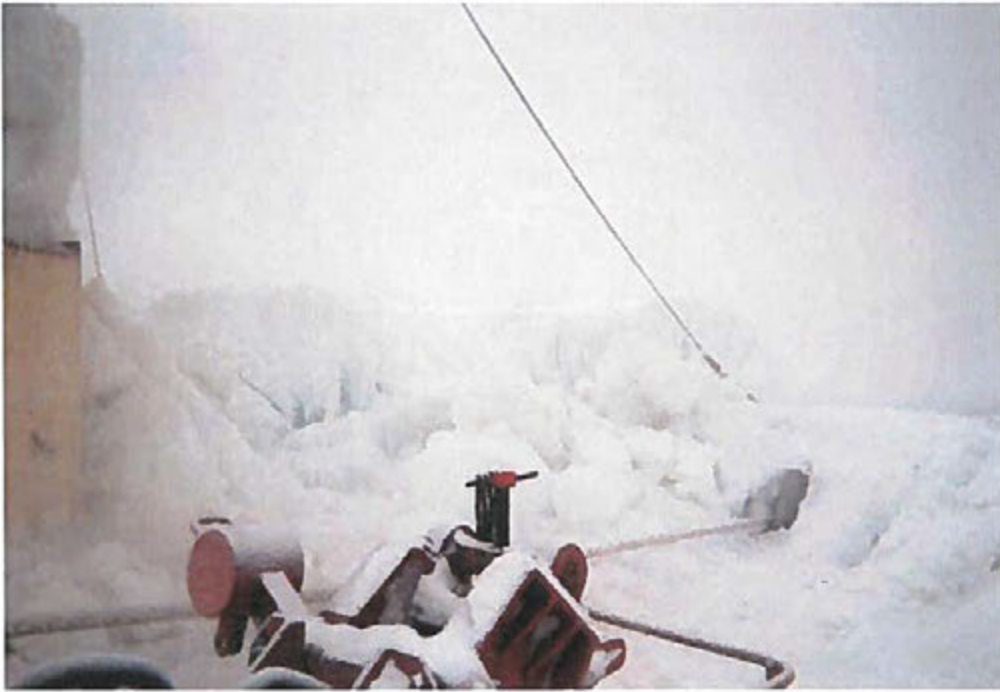
Figures 5.3I– Guy wire view after de-icing
