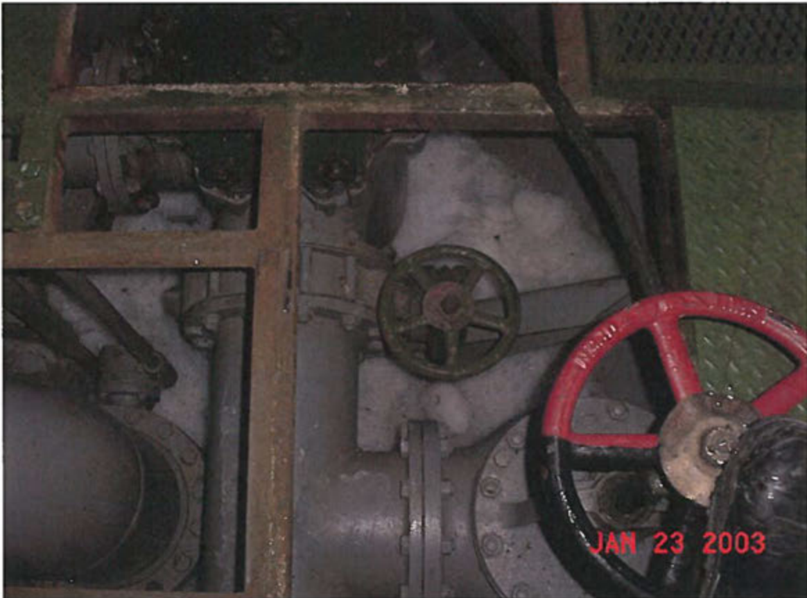
Figures 3.7A – Frazil ice accumulation at the bottom of engine-room bilges after numerous seawater strainer cleaning
