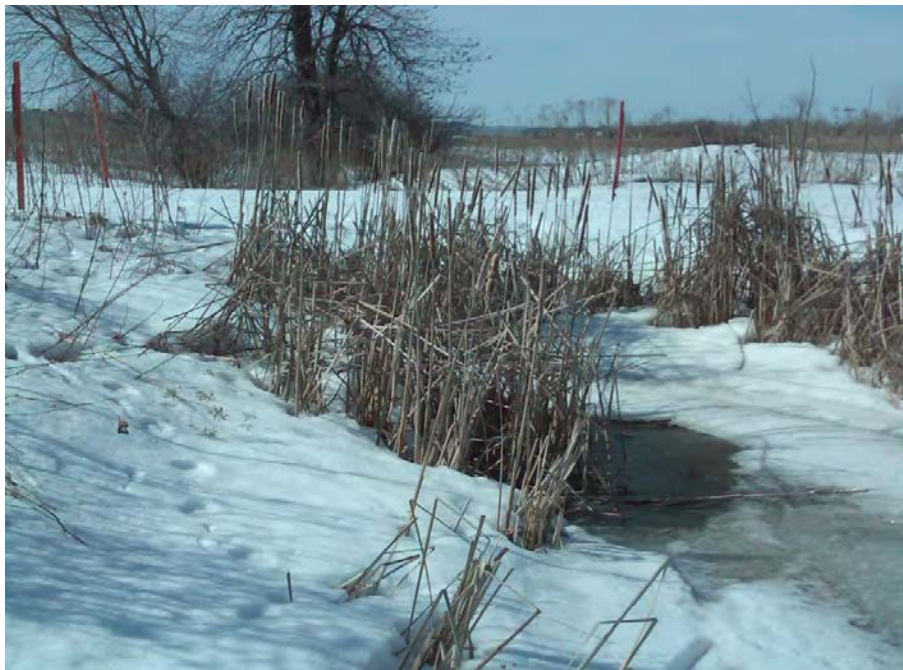
Figure 18: Partial view of a culvert and watercourse observed in the portion of the Site consisting of vacant lots located on the north side of F.X. Tessier Street. View toward the west.
