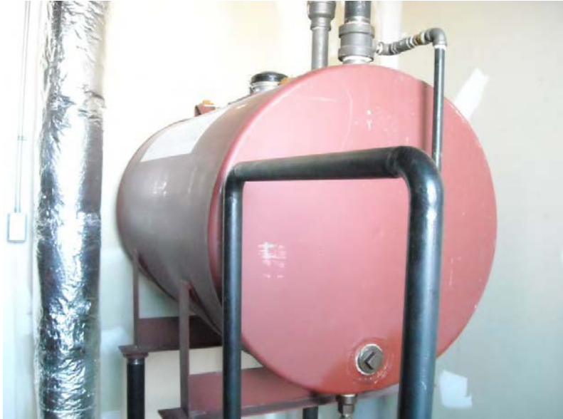
Figure 7: Partial view of the double-wall diesel AST associated with the sprinkler system, 3600 F.X. Tessier Street building.
