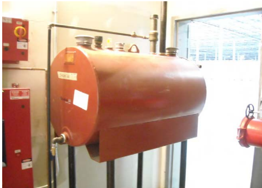
Figure 11: Partial view of the double-wall diesel AST associated with the sprinkler system (400 Marie-Curie Street).
