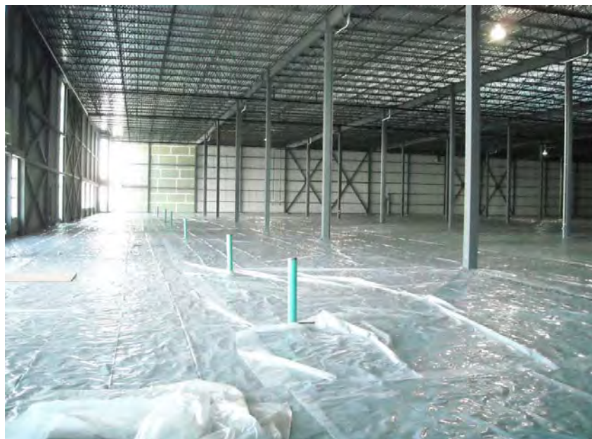
Figure 10: Partial view of the inside of the vacant and unfinished Site building located at 400 Marie-Curie Street.
