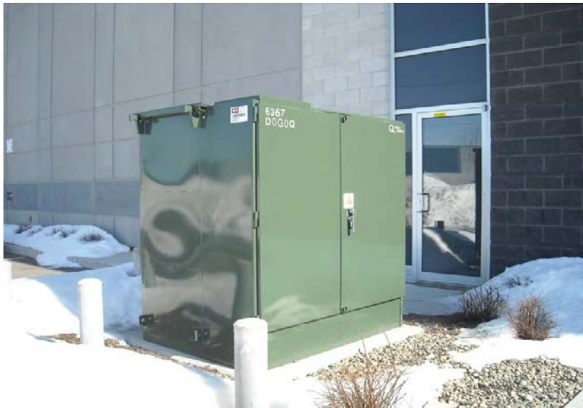
Figure 9: Partial view of the transformer located in front of the 400 Marie-Curie Street Site building.
