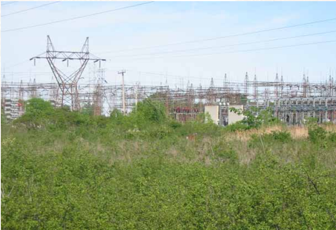
Poste Hydro (C)
