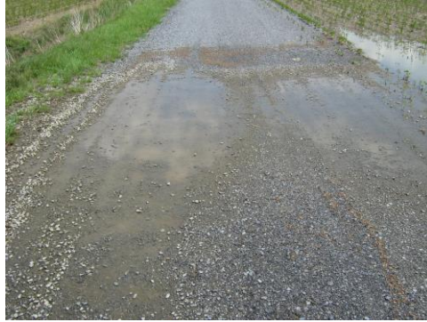
Poor Runway Surface Condition South Threshold looking North
