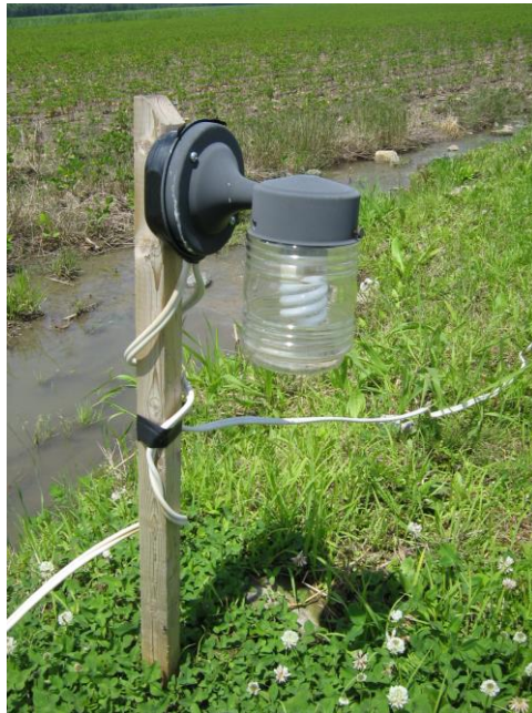
Typical Light Marker North of Runway Mid-Point
