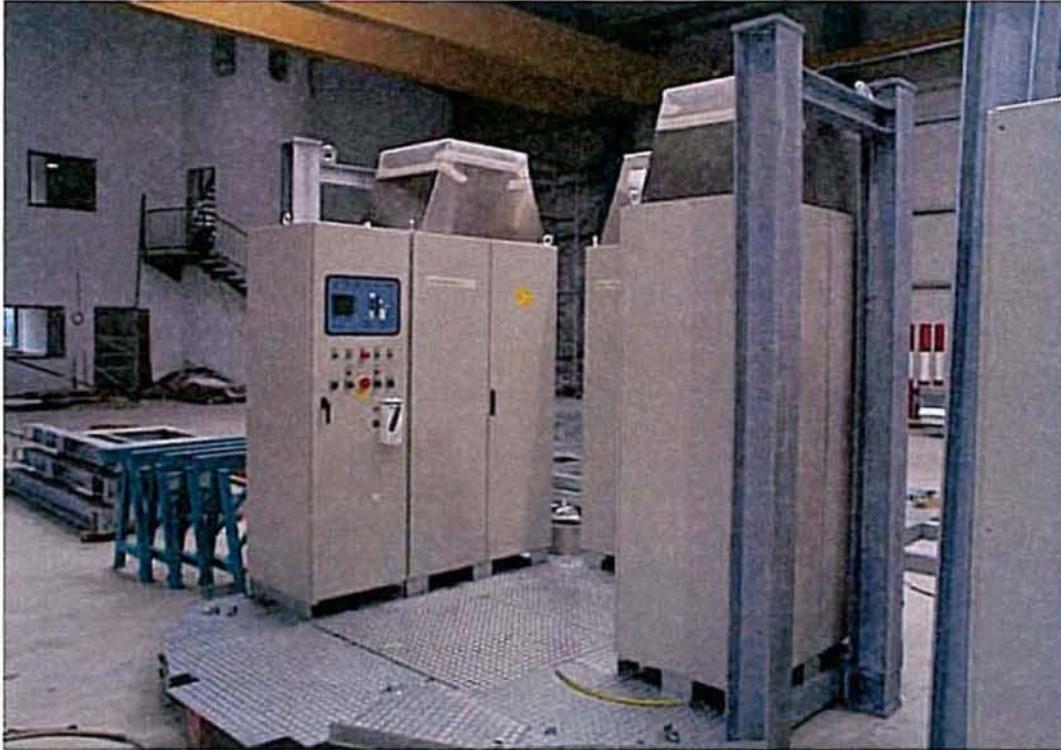
Figure 5 – Control panel and power cabinets are installed on medium level
