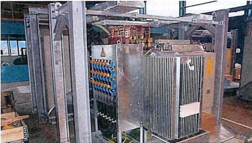
Figure 4 – Circuit breaker, switchgear and transformer installed.
