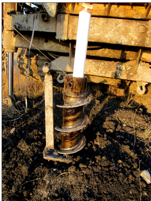
Photo 17: View of the hollow stem auger smeared with free product, at monitoring well location MW-12-162.
