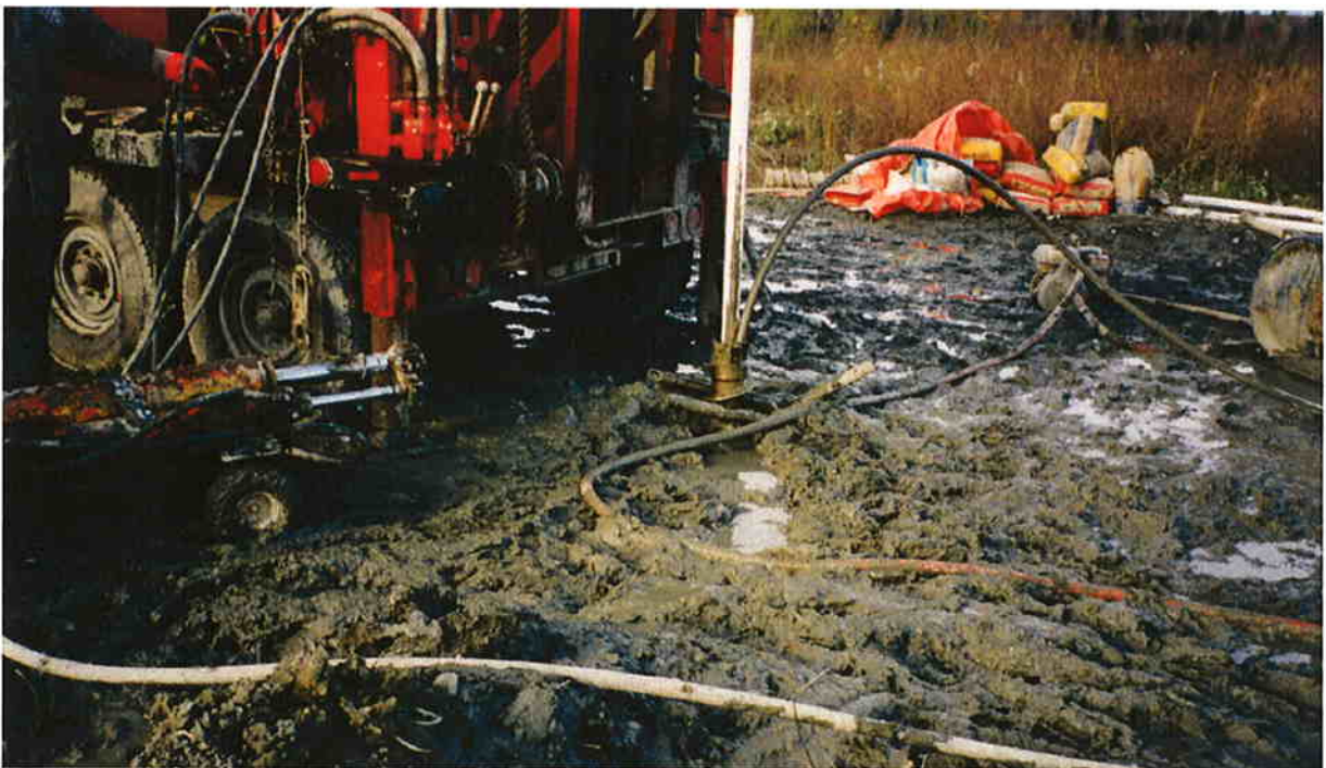
2. Injection du coulis ciment-bentonite au puits PO-03-01C / Injection of cement-bentonite grout at well PO-03-01C
