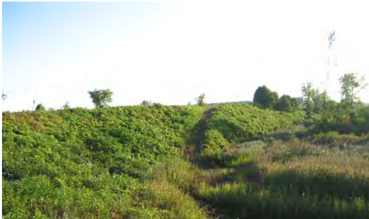
Figure 2: Downstream slope before vegetation control
