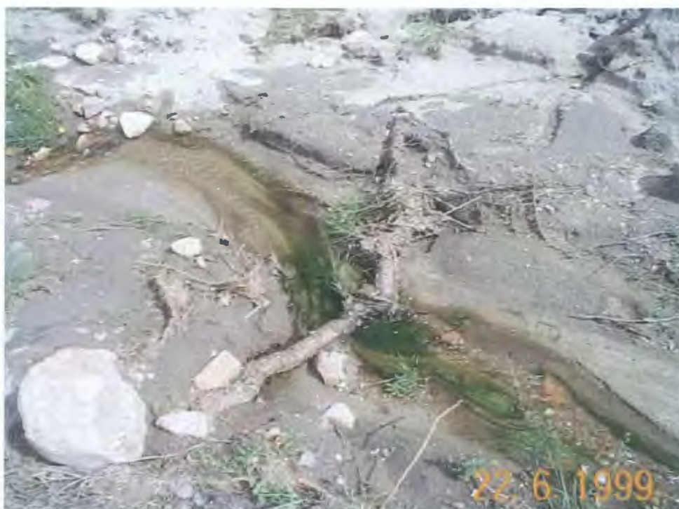
Figure 3. Large pine root located in the channel of the breach opening of a failed Air Force Academy waste lagoon pond dam (David Eyre, Senior Civil Engineer, Air Force Academy, Colorado, 1999).
