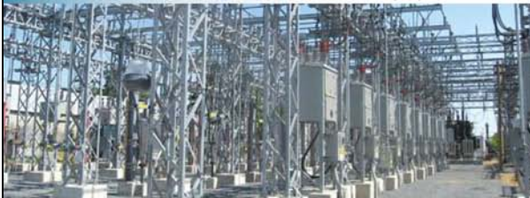
An example of a 25-kV side, located at Saint-Maxime substation in the borough of Saint-Hubert.
