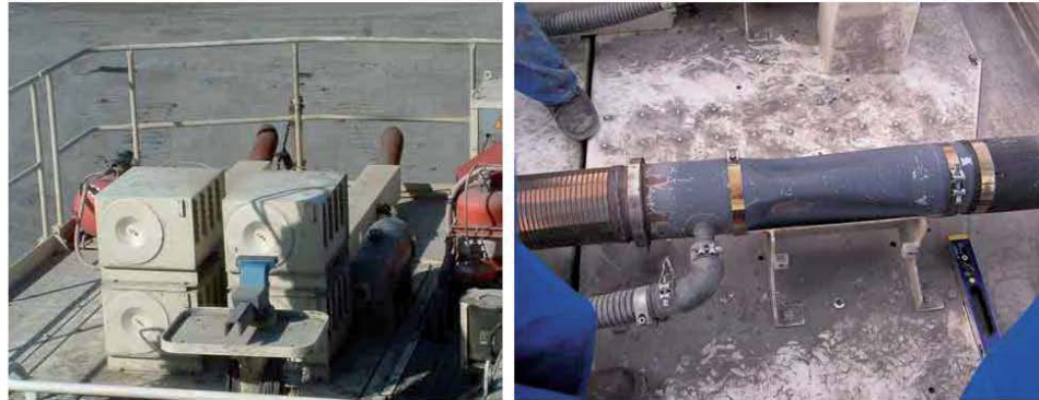
Figure 4: Engine air intake filters and exhaust venturis.
