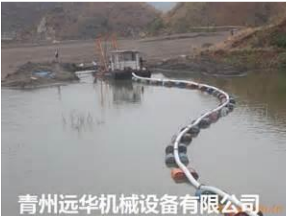
Figure 16: Photo of spoils discharge pipe from dredge
