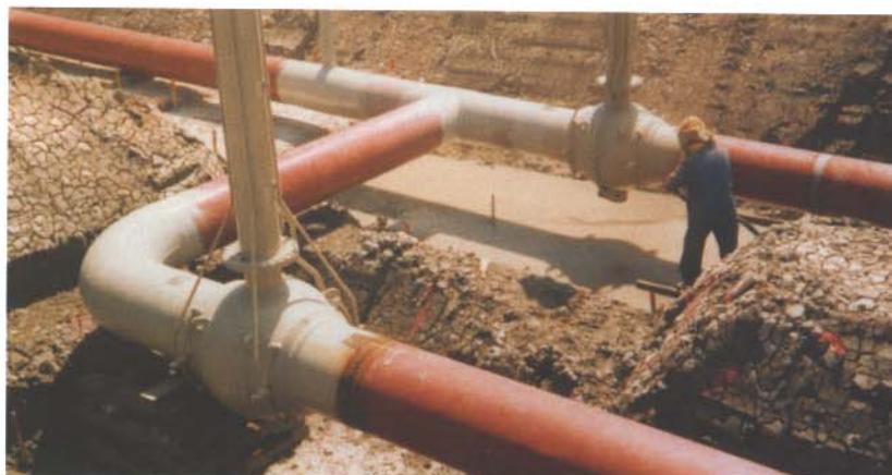
TRANSCANADA PIPELINES LTD., Saint-Lazare
