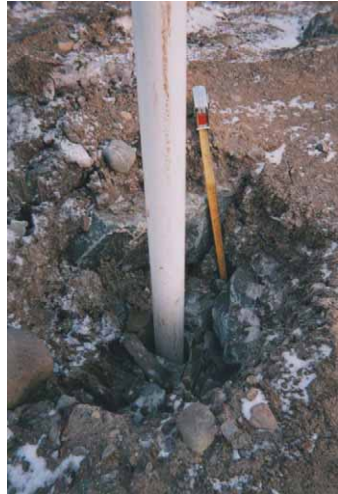
Photo 9. Close-up of borehole BH-5. Note fill placed around blasted rock layer that covers the foot print of tank T-101. Borehole was drilled through blasted rock and continued to a depth of 15m for boreholes BH-5 and BH-6 and 30m for HQ (75mm) borehole BH-7.
