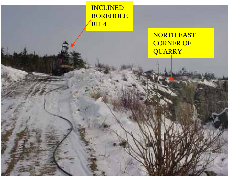
Photo 4. Location of inclined borehole BH-4 (during drilling). Drill is directed perpendicular to the fracture plane in order to intercept a continuation of the plane below tank T-100. Other than minor deformation features caused by folding of the rock in the geological past, no indications of the fracture plane were observed in the core of borehole BH-4. Borehole BH-4 revealed solid sandstone below the elevation of tank T-100.
