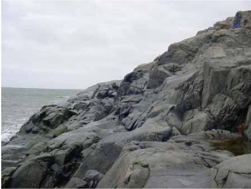
Photo 18. Looking east. Vertical and sub-vertical jointing striking parallel and perpendicular to shoreline. No low dipping beds or seams were observed on the upper portion of the beach above the high tide line that may interfere with the foundation further to the south.
