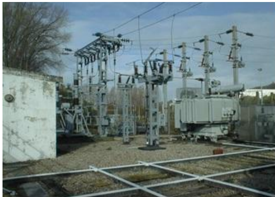
Figure 8 Sous-station 25kV de Soquence – France
